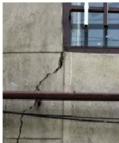
Fig. 2. Example of wall cracking and structural damage in an existing building caused by differential settlement due to adjacent construction.
