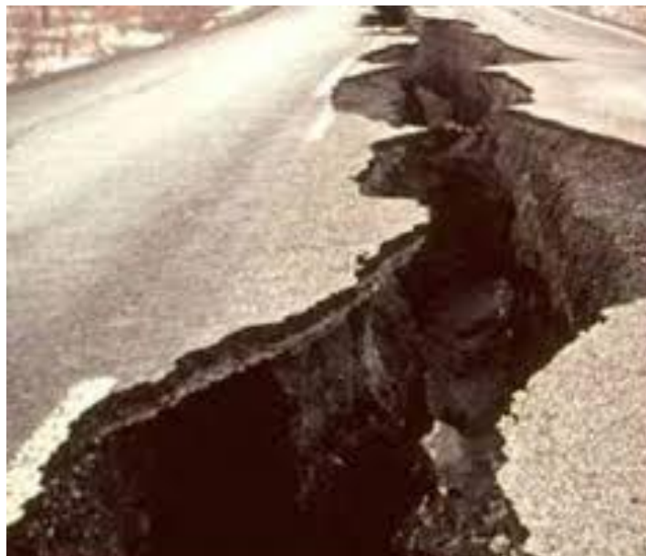
Fig. 7. Longitudinal cracking in a road embankment during the Peru earthquake, reflecting tensile stresses along the road axis.
