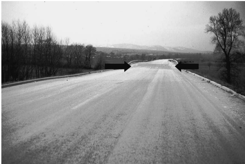
Fig. 3. Permanent embankment displacements near an overpass caused by the 1980 Irpinia earthquake, Lioni, Italy.
