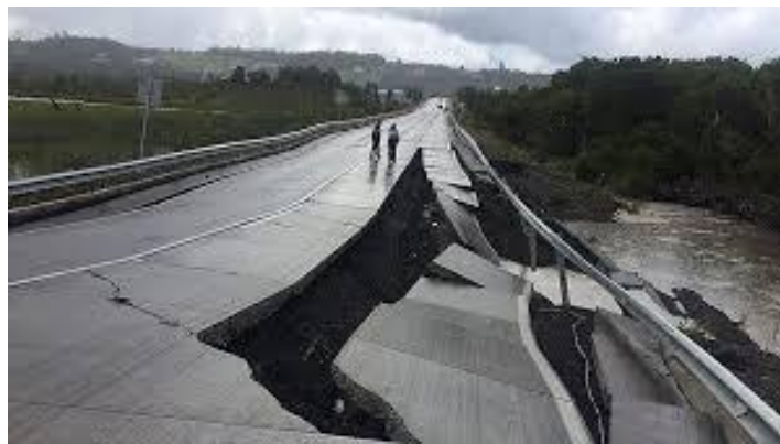
Fig. 6. Shear failure in a road embankment during the 2010 Chile earthquake, showing notable lateral pavement displacement.
